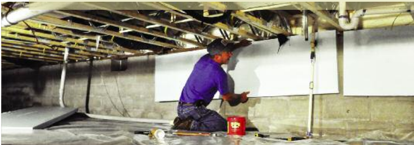
Co-op members enjoy energy-efficiency benefits through a home weatherization program carried out through Hoosier Energy and its member cooperatives.
